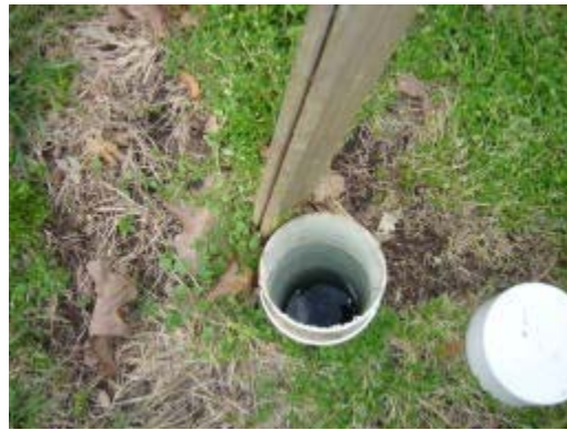
Chamber system full with septic effluent
